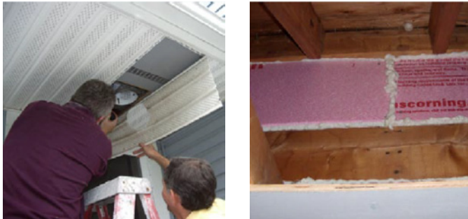
Figure 10. When researchers pulled back the porch ceiling, they found the wall board was missing so nothing was covering the insulation on this exterior wall. An air barrier of rigid foam board was put in place with spray foam (Image: Moriarta 2008).
